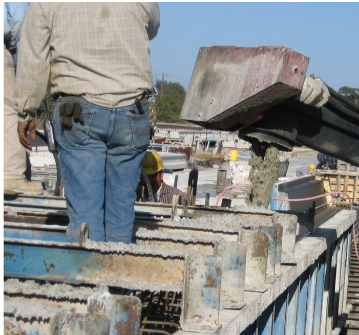
Figure 3.34 Filling the webs and end blocks around the interior-void form, held in place with hangers
